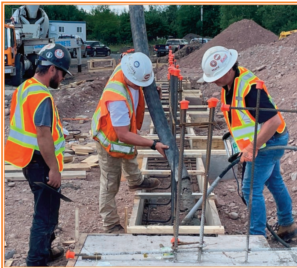
Crews with Iron Maple Constructors pour the footings for the new $6.1-million fire station in Springhill. The new facility, which is expected to be completed in late spring 2025, will replace the existing Springhill fire station and serve as one of four hubs within the municipality. (Darrell Cole - Municipality of Cumberland photo)
