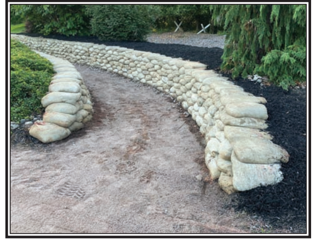
Good for at least 15 more years, the trench at Veteran's Memorial Park received 1100 bags containing 19 cubic yards of concrete from Easy Concrete. A team of over 50 volunteers started unloading the first truck at 8 am, and by 1pm had emptied the second truck. (John Gilley Photo)
