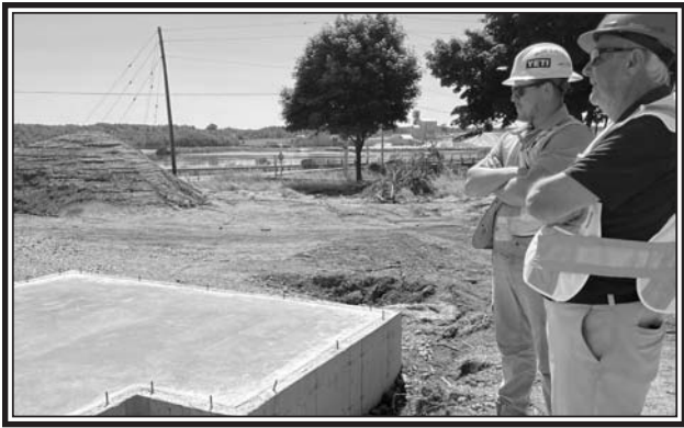
Dylan MacIsaac (left) of Iron Maple Constructors and Pugwash Library project lead Roger MacIsaac look over the newly poured concrete. (Darrell Cole Photo)
