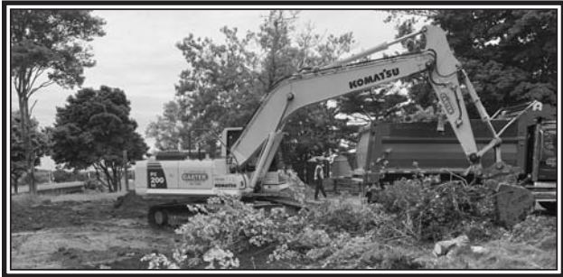
Excavating work at the beginning of the project on the corner of Highway 6 and Durham Street in Pugwash. The new library will be completed by the end of October. Roger MacIsaac/Municipality of the County of Cumberland. (Darrell Cole Photo)
