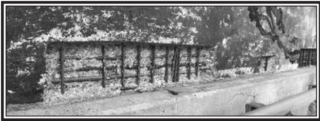
Some areas of the Gosse deck needed repairs. Workers have chipped out certain areas reading the deck to receive a new weatherproof membrane prior to final paving. (Submitted)
