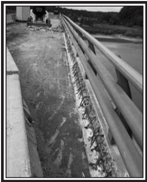
The asphalt surface and curb face have been jack-hammered out to expose decking rebar during the rehabilitation work. (Submitted)
