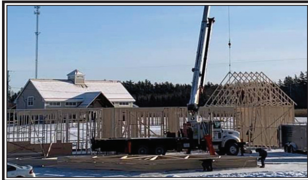
Davey Green Construction was busy working on the new Pharmacy throughout the winter, with roof trusses added back in December.
