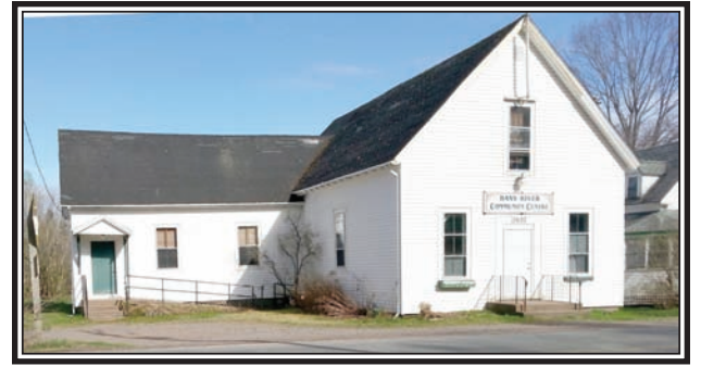
Bass River's Victoria Hall is raising money for a new roof and other upgrades.
