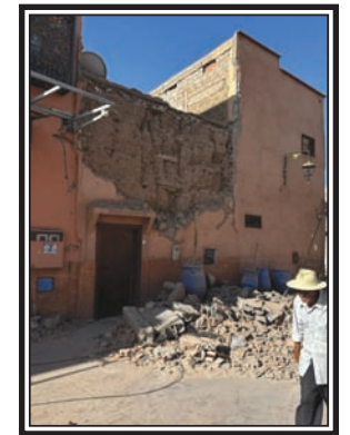
Damaged but still standing, Marrakesh. (Submitted)
