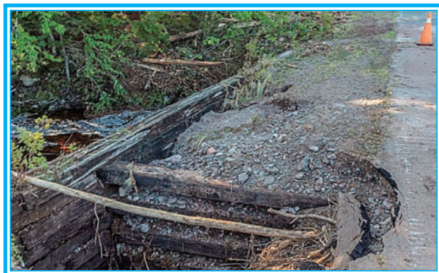
Heavy runoff exposed an old wooden crib. It will take a while to correct all the damage from the August 29th storm. (Lawrence R. Nicoll Photo)
