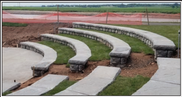
The seating has been finished and sod installed between the rows of seats in the amphitheatre. (Contributed)
