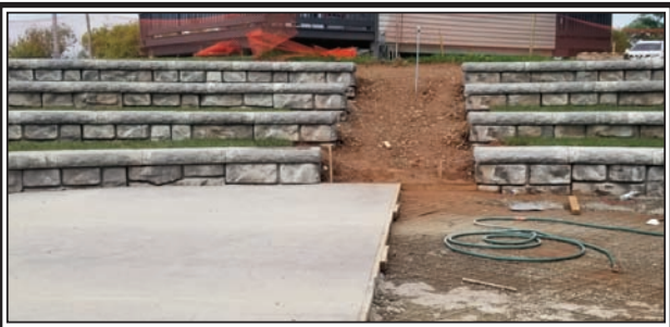
Nearly half of the amphitheatre floor has been poured and finished. In future many entertainment acts will be entertaining visitors in the curved seating. (Contributed)
