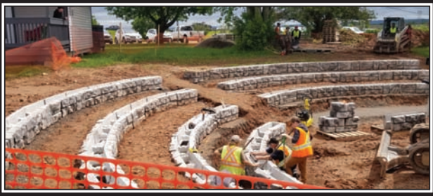
Workers check the levels for the curved seating in the amphitheatre area of the Fundy Discovery Site, which was officially opened on September 21. Supplied by DuraCast, Dartmouth the pre-cast boxes and filled then seating is installed. (Contributed)
