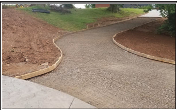
The rebar and border forms have been put in place awaiting for a concrete pour. A portion of the walkway has been installed in the upper corner. (Contributed)
