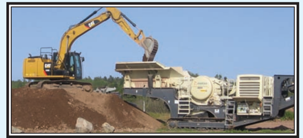
You have to work fast to keep the hopper in the screener filled for the sewer pipe contract being performed by Dora Construction. (Rees Photo)
