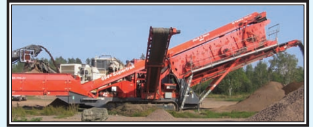
Several workers are required to screen, crush and stockpile gravel to be used when laying new sewer pipes in Parrsboro. (Rees Photo)
