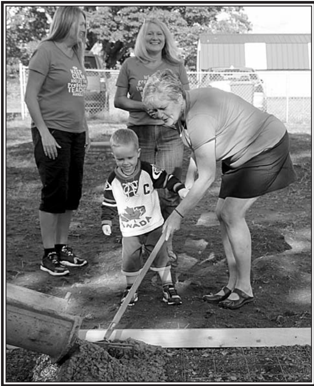
Lower Onslow Preschool teacher Joann Michelin helps Connor Roberts Moore spread the cement to make a pad for a picnic table, as fellow teachers Claire Shepherd and Shannon Smith look on. A new playground is being built at the Lower Onslow Community Centre. (Harrington Photo)
