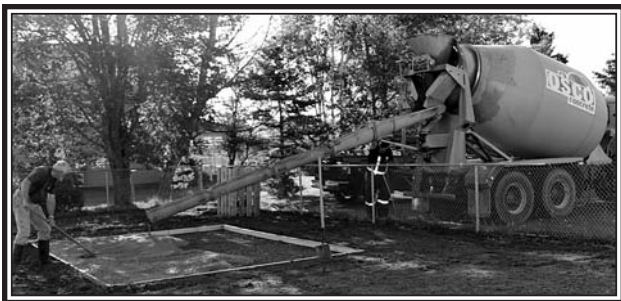
Volunteer John McKay makes sure the cement is level as work begins on the new Lower Onslow Community Centre Playground. Kerby Wallace, of Glenholme Ready Mix delivered the donated cement to Lower Onslow. (Harrington Photo)
