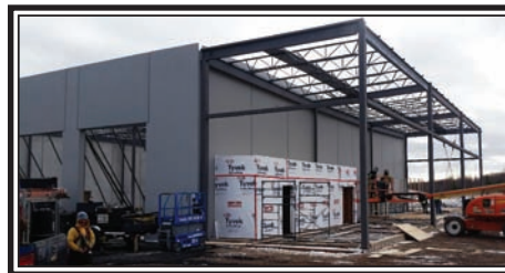
Most of the East Coast International building in the Truro Power centre was built with tilt-up pre-cast concrete panels but an additional bay was required with plenty of separate ventilation for cutting and welding, and similar work. This additional bay was built with traditional structural steel frame. RKO Steel, Dartmouth supplied the structural steel for the entire building. (Submitted)
