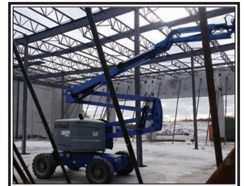
RKO Steel, Dartmouth supplied the structural steel requirements for the East Coast International new building at the Truro Power Centre. (Submitted)
