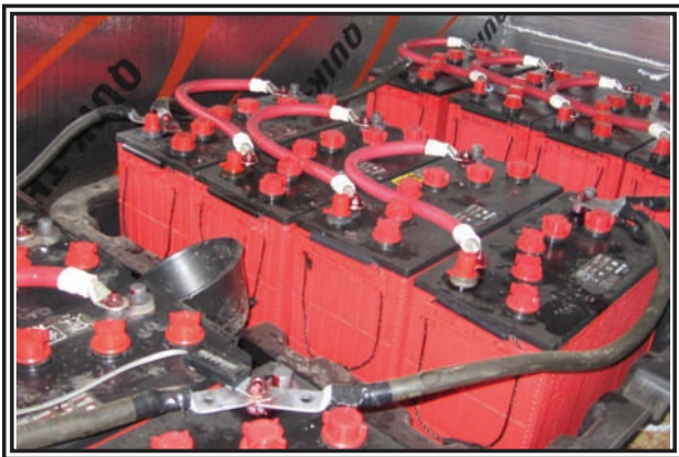
These 12 - 12v batteries provide sufficient storage for evenings to operate the household appliances, which includes television, computers, lights, two refrigerators, two deep freezers and washer. Propane is used for heating, dryer, stove and oven. (Rees Photo)
