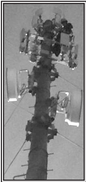
There's a lot of equipment on top of a communications tower.
