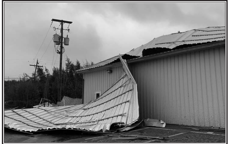
The steel roof on the Masstown Market bakery building peeled right off during hurricane Fiona. (Harrington Photo)
