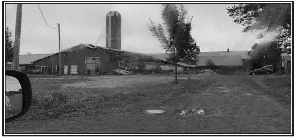
Several barns in the area had damage, including this one in Central Onslow. (Harrington Photo)
