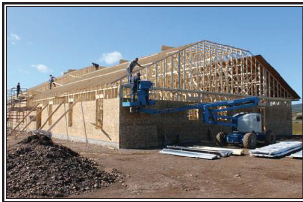
Immediately after the walls were up the rafters were installed and volunteer workers started installing sheathing for the roof. (Submitted)
