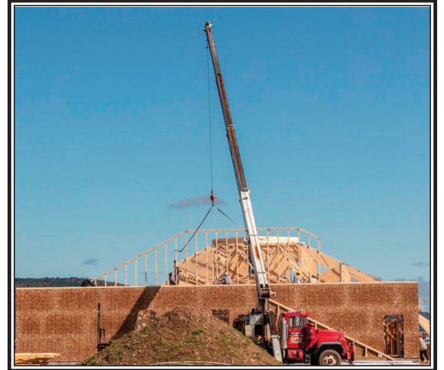
A crane lists rafters for the Open Arms Church construction in Parrsboro recently. In typical "barn raising" fashion an army of volunteers had the walls up and roof closed-in in five days. An incredible monument to what work can be accomplished when the need arises. (Lawrence R Nicoll Photo)
