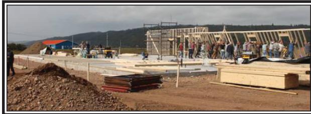
In traditional barn raising style numerous workers are required to raise and secure the walls of the new church. (Submitted)
