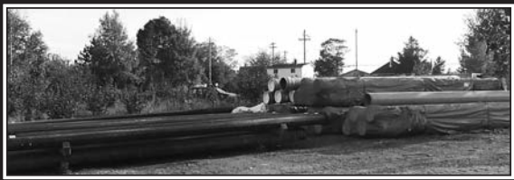
This is just a small portion of pipe in the marshalling yard awaiting burial throughout Parrsboro. (Rees Photo)
