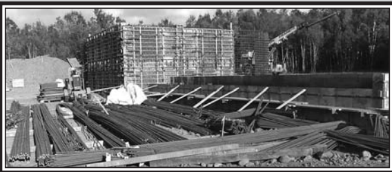
There's lots of rebar, on-site, awaiting for construction workers to set in place for the wastewater treatment plant. Concrete forms ranging from four feet to sixteen feet high will form the walls of Parrsboro's new wastewater treatment plant being build by Dora Construction. A 120 metre pour was scheduled for September 28th to be followed by another 70 metre pour on Friday, September 29th. (Rees Photo)
