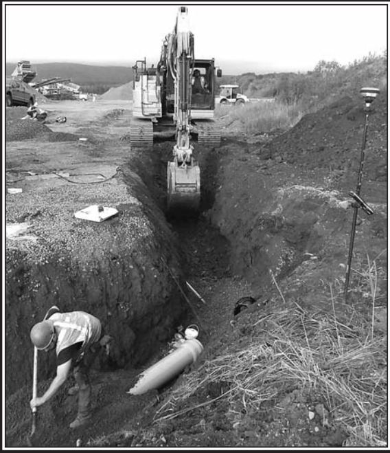
Brycon Construction hired Dexter's to install the main collector line from the Abitoeau into the Wastewater treatment plant under construction by Dora. (Rees Photo)
