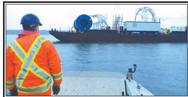
An unidentified crew member on a safety boat keeps watch as the barge containing FORCE's underwater cable passes by. The second cable was installed in Minas Passage on Sunday, October 21 st . (Submitted)
