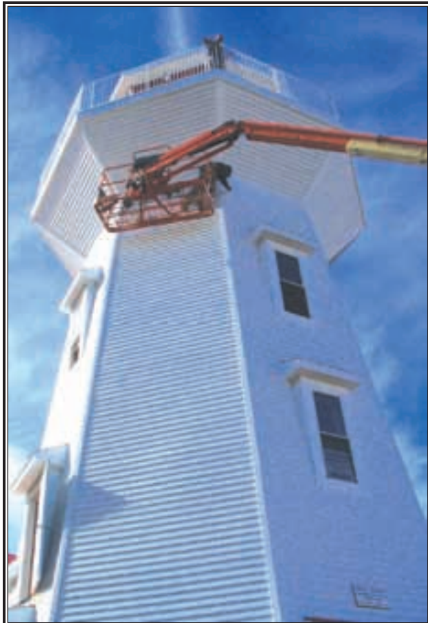
It's long way up. The lighthouse at Masstown Market, in its own way, has become an icon. Rushing to complete exterior construction, before winters frigid weather, workers paint the exterior of the lighthouse, which will house a fish market. (Feetham Photo)
