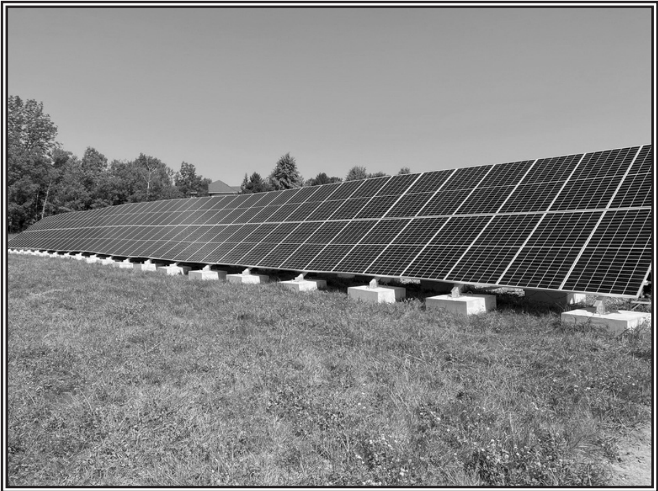
The Windsor Elms Village solar farm - another LMMW group project. Photo courtesy of LMMW Group.
