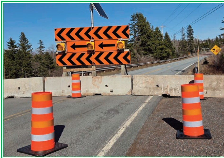
The Lower Portapique Bridge on Trunk 2 is closed for repairs until further notice. Tom Taggart, MLA advised the Shoreline Journal shortly after lunch on April 1st that the bridge was undergoing a detailed inspection and it was expected it would be closed. This photo taken at entrance to Joy Laking Art Gallery shows the detour barricade. The detours are East Montrose Road and West Montrose Road adding about 10 minutes to travel on Hwy 2. For detailed explanation on bridge replacement, please see Tom Taggart's column on Page 5. (Rees Photo)
