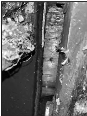
These two photos show the damage to the new baler when the flange that attaches the side ram got torn away from the main baling chamber. This happened due to poor factory welds and the repair was done through warranty with only one week of down time. (Contributed)
