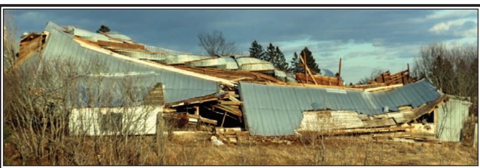
Power of the wind! Mother nature huffed and puffed and down came this barn on Staples Brook Road, Debert. (Harrington Photo)
