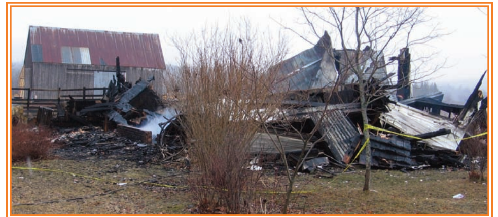
This is all that remains of the large farmhouse belonging to Carolyn Cooper, Five Islands, which burned on evening of Friday, March 25th. The charred remains were still emitting some smoke on Tuesday, March 29th, four days later. (Rees Photo)
