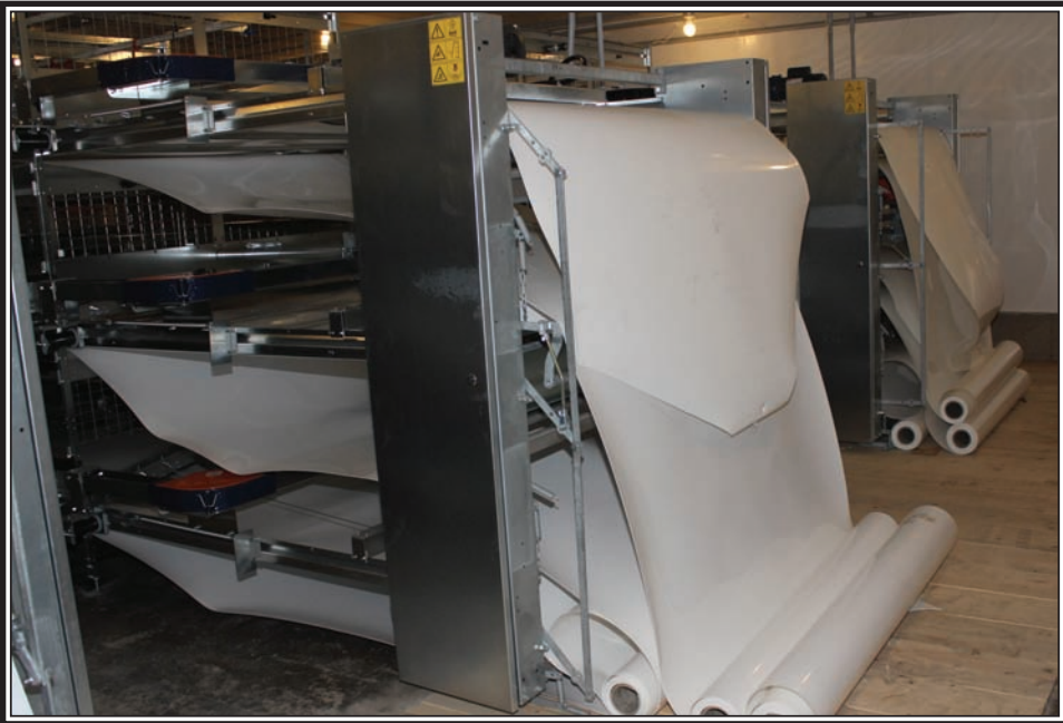
The automated manure removal system will see these white collection rolls run by a 24" inch conveyor belt, supplied by Northumberland Silos.
