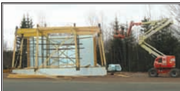
Construction is underway at the Masstown Market for a new Lighthouse and Fish Market. The lighthouse will offer a towering view of the surrounding area when completed. (Harrington Photo)
