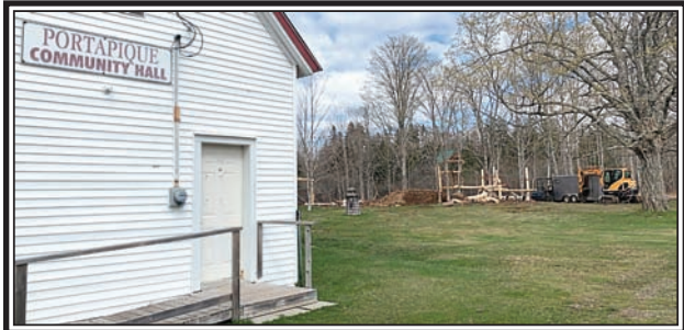
The new playground at the Portapique Community Hall build-up site is under construction, Completion is tentatively planned for end of June. (Submitted)
