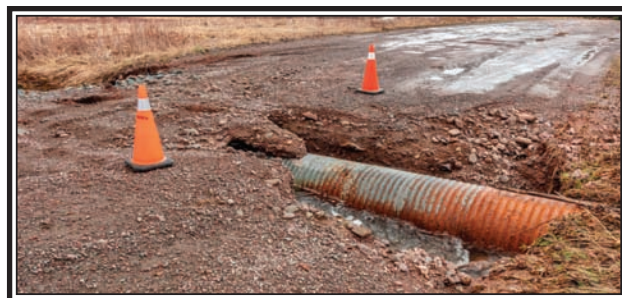
Heavy rains in late April caused extensive damage to several sections of Fox River Road. The road was nearly impassible, when this culvert was almost totally exposed. (Lawrence R Nicoll Photo)
