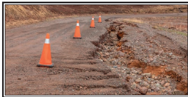
Nova Scotia Transportation & Infrastructure employees spent many hours delivering and placing highway detour cones to mark the dangers area on the rural roads following heavy rains. This picture shows some of the damage on Fox River Road. (Lawrence R Nicoll Photo)
