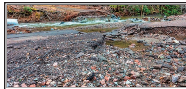
A portion of Smith Hollow Road was completely washed out during the damaging rain storm. The heavy surge of water deposited the culvert on the far left in this photo. (Lawrence R Nicoll Photo)
