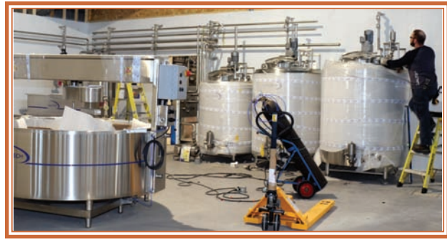
Qualtech custom designed the milk pasteurization equipment to fit within the Masstown Creamery space. To the left is the Qualtech cheese vat.
