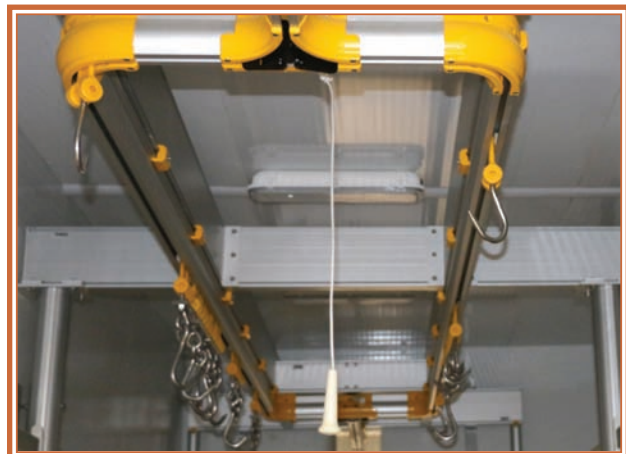
A sectional overhead rail system will be used for hanging up, transporting and storing meat inside one of the walk-in refrigerators of Masstown Butcher Shop.
