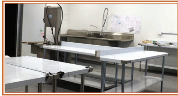
One of the meat saws and several stainless-steel butcher tables have been installed in Masstown Butcher Shop.
