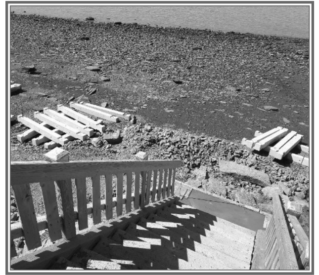
The Joggins Fossil Institute has new platform and aluminum stairway to the Cliffs. Constructed in April and May, this more stable infrastructure will, hopefully, stand up to the winter weather served up by the tides, wind and ice of the Cumberland basin. Municipality of the County of Cumberland made the stairway possible. (Submitted)
