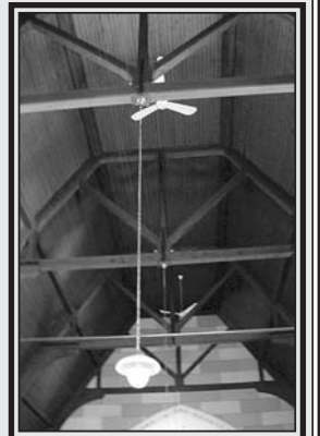
The roof of the Saint James United Church was built like the hull of a ship.
