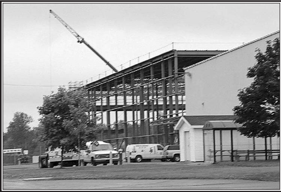
Construction on Phase One the 236,000 square foot expansion is moving right along, providing construction jobs totalling up to 200. (Harrington Photo)
