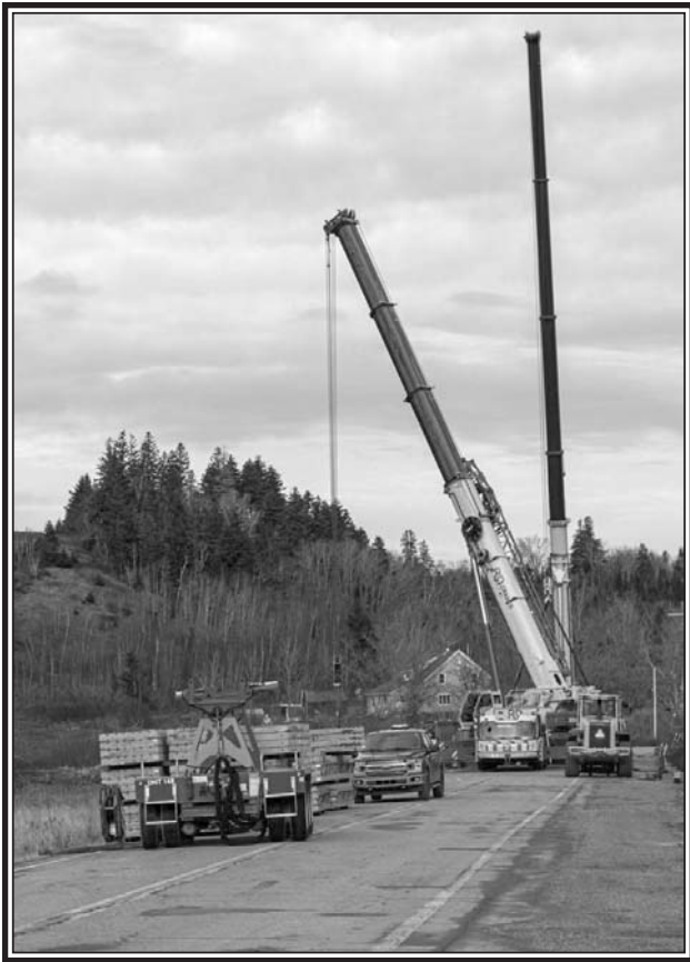
The bridge repair on Hwy 2 at Cannan/Harrison Settlement Rd was finally able to proceed. On November 28, cranes were pulled from other jobs and the bridge lifted into place. The bridge opened on Monday, December 11th. (Lawrence R Nicoll Photo)
