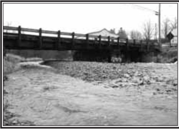
The build up of gravel under the bridge in Bass River has area residents concerned there could be damage to the bridge or flooding this winter. (Harrington Photo)
