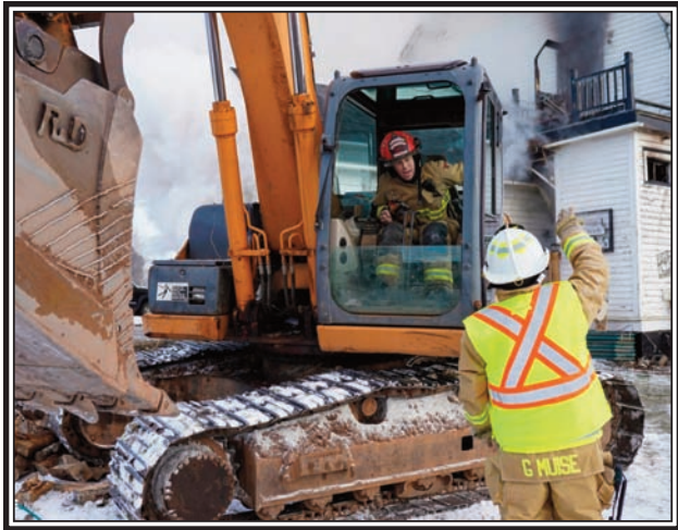
Blayne Turner of OBFB put his construction experience to work knocking down the fire.
