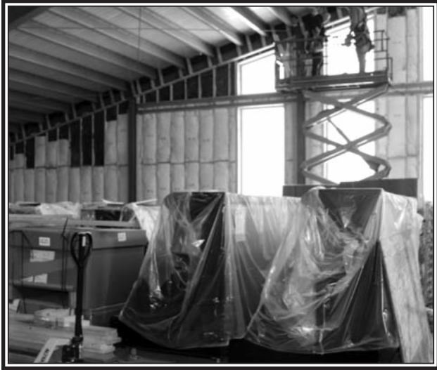
Masstown Butcher and Dairy - the outside of the new building has looked near completion for several weeks, even the parking lot is paved. Inside there is a flurry of activity, as dozens of skilled workers continue with the installation of walls, floors and specialized equipment. Scattered throughout this Shoreline Journal are a series of pictures taken on January 23rd. Above, work continues at the front entrance to the new building. A few of the display cases can be seen in the foreground. (Harrington Photo)
