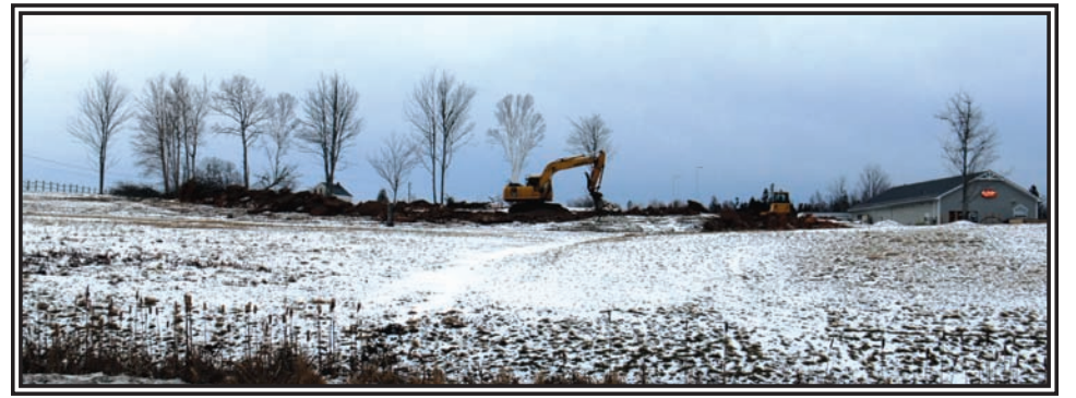
Culgin Construction have started excavating for a new 15,000 sq ft building across the road from Masstown Market adjacent to Masstown Petro-Canada. The building will be used for a butcher shop, dairy and cheese making operation. (Rees Photo)
