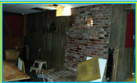
A brick fireplace, located in the basement pub has seen better days.
