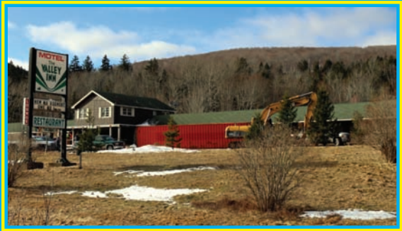
A demolition sale was held at the Valley Inn, Wentworth on Saturday, Jan. 28th. An excavator was already on site to begin the tear down.
