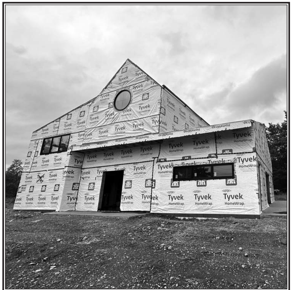
Work continues on the Portapique Community Hall, which will be a lovely permanent location for the weekly Farm Market.
