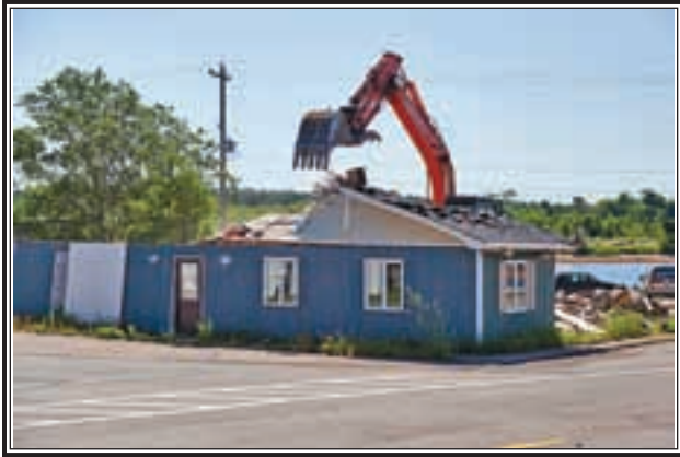
July 9th a sad chapter in Parrsboro when what was once Berry's Restaurant was demolished. In the family since the 40's when it started as a coal and ice delivery business, and sharpened skates for the many who skated on the Aboiteau. Ravished by fire in 2010 and vandalism, it's time had come, and gone. (Lawrence R. Nicoll Photo)
