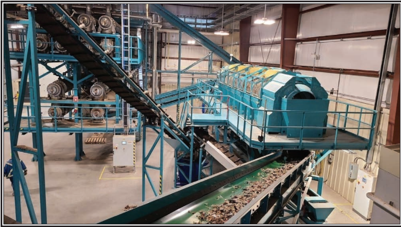
Conveyor belts at work in Sustane's fully-automated "repurposing" facility in the District of Chester. Photo courtesy of Kevin Cameron.
