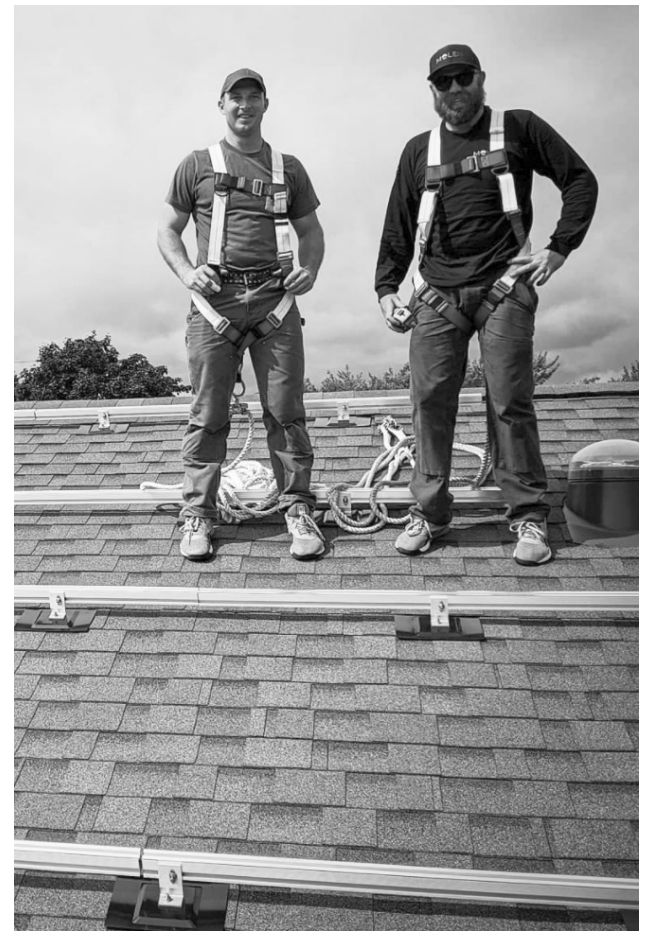
Molen Services installation professionals, Peter MacGillivray, left, and Kyle Chisholm are shown during the installation of rooftop panels. (Submitted)
