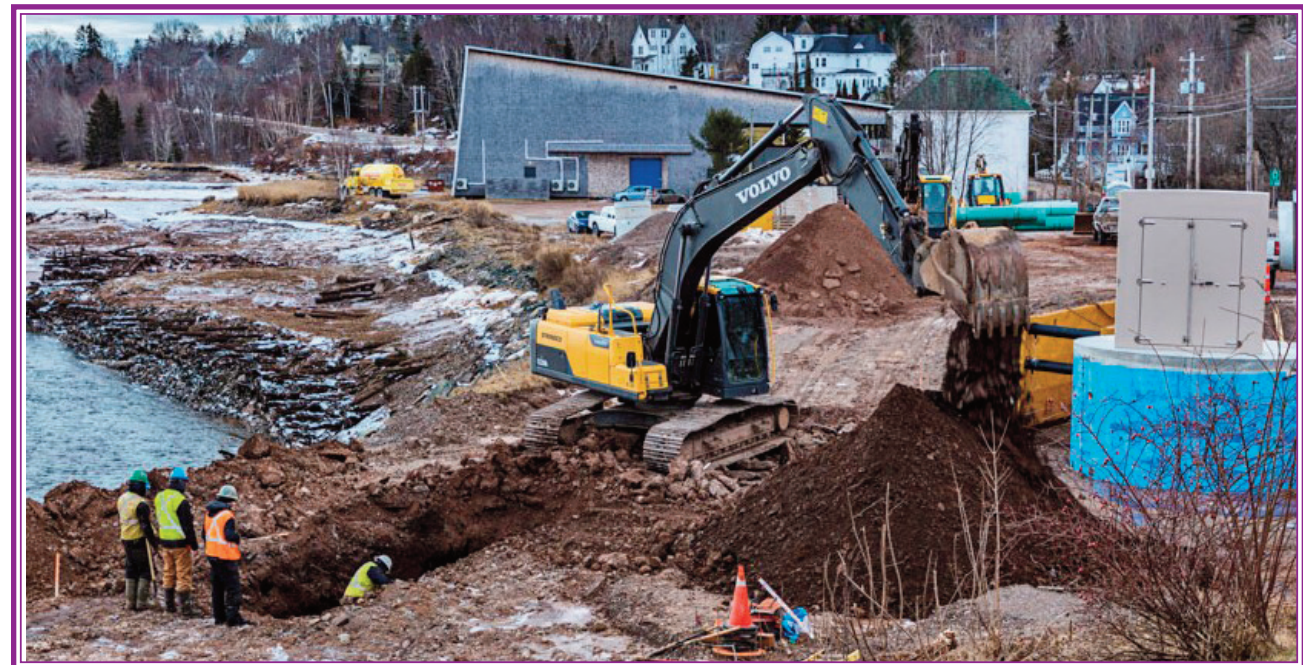
Workers installing sewage line with Ships Company Theatre in the background. (Lawrence R. Nicoll Photo)
