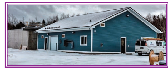
The new sewage treatment plant shown above is still undergoing construction. (Lawrence R. Nicoll Photo)
