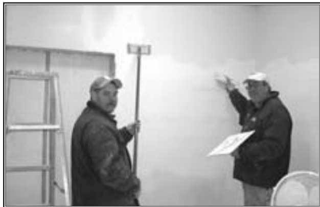
Contractor Aaron Smith (right) and Greg Singer work on dry wall finishing in the washroom at the Debert Military Museum. (Harrington Photo)
