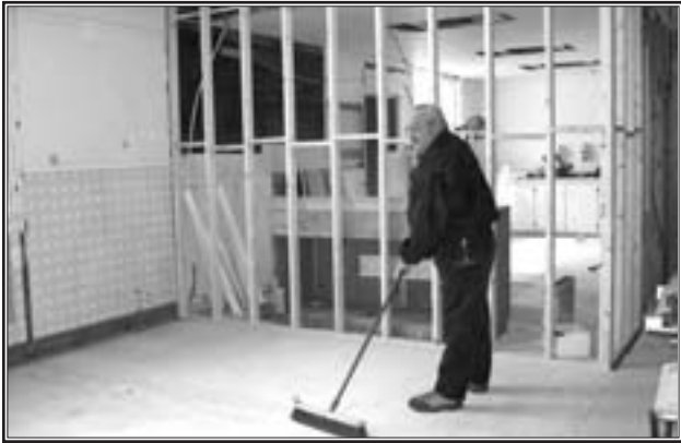
Past President of the Debert Military Museum, Mike Taylor, sweeps up a bit of dust from the new subfloor at the Museum. Renovations are taking place throughout the Museum, including this kitchen area. (Harrington Photo)
